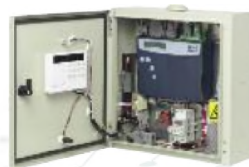
Squirrel 2020 in an electrical enclosure
